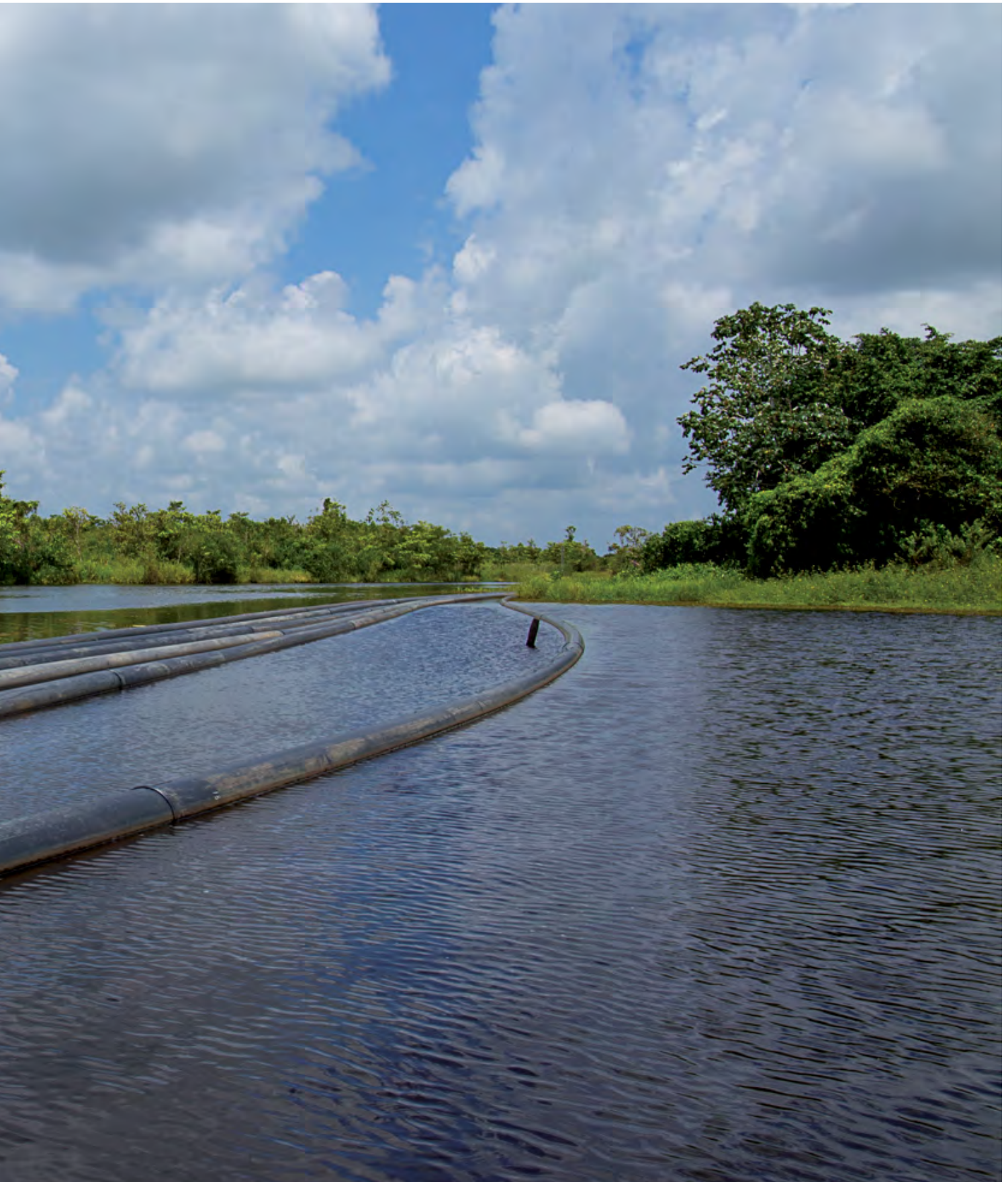
■ Pipelines in the wetlands to transport the crude from well to treatment plant.
