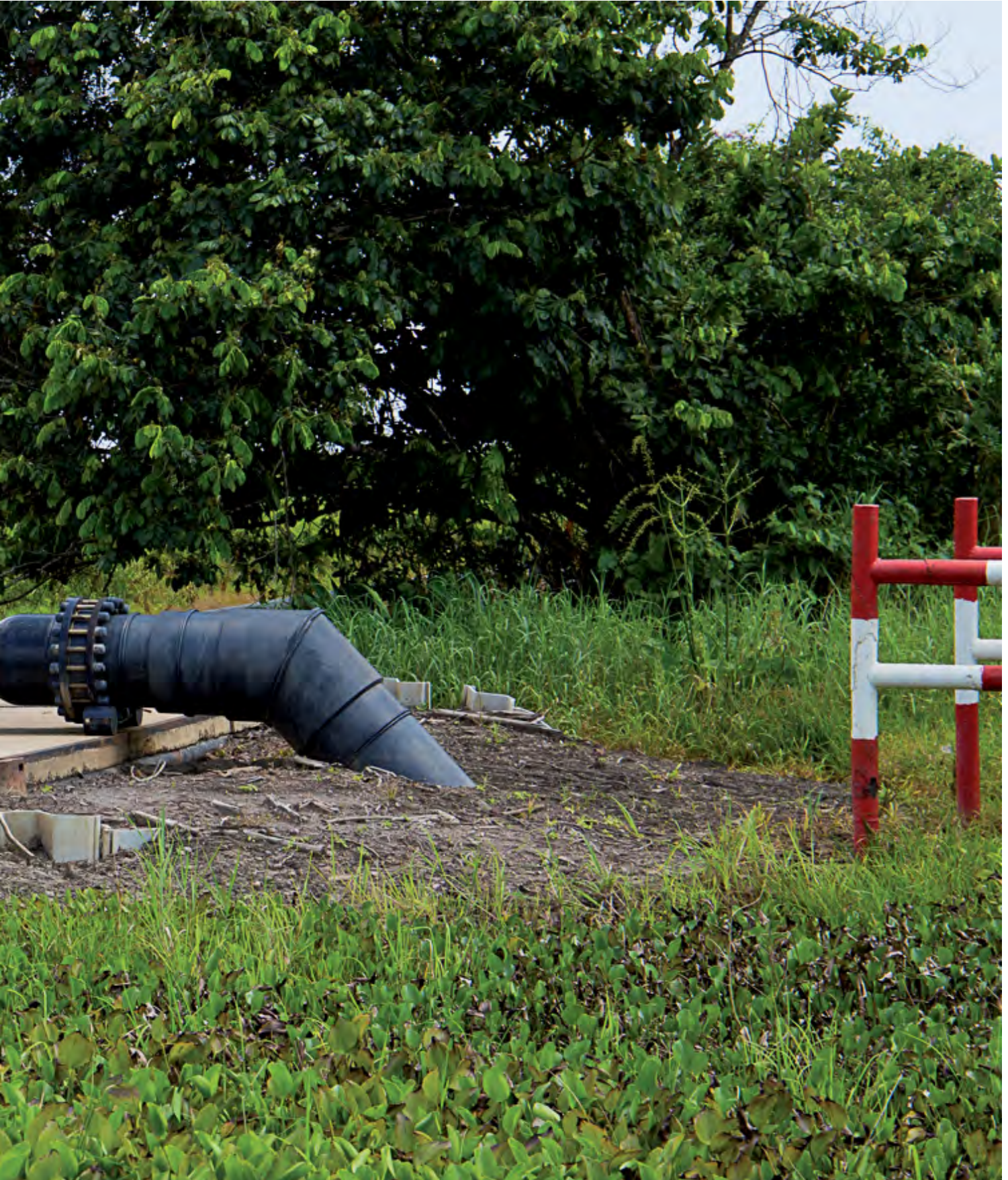
■ Pipeline in the oilfield.
