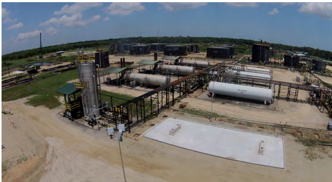
■ Crude treatment plant TA58 in Saramacca.
